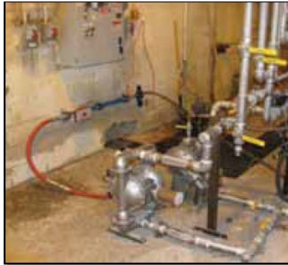
Grains and Powders Manufacturing Facility Saint Gobain • Niagara Falls, NY
